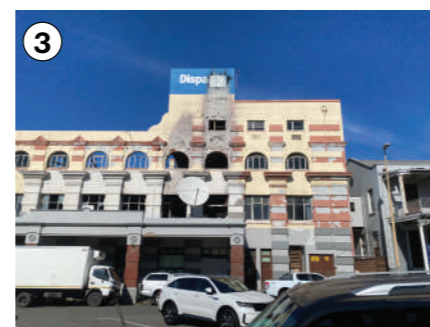
Figure 27 : The Daily Dispatch building, damaged by fire and gradual decay. Source: Author (2023)
