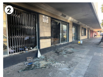
Figure 26 : Ground-floor vacant commercial spaces marred by vandalism. Source: Author (2023)
