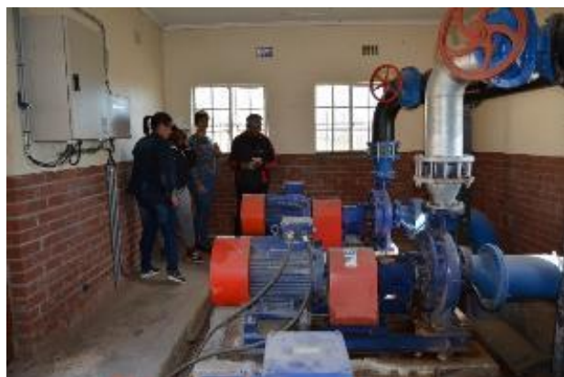
Figure 27: Site visit with CRAs and municipal representative exploring Noordhoek's water system. (Source: Author's own)
