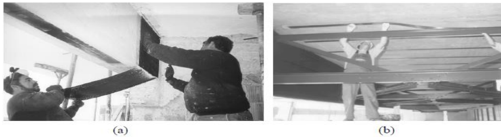
Figure 2.15. (a) Hand lay-up of CFRP sheets or fabrics, (b) Application of prefabricated FRP strips (FIB, 2001).
