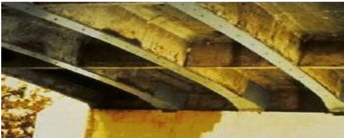
Figure 2.8. Typical steel plate bonding for flexural strengthening RC beams of a RC bridge (Alkhrdaji, 2013).
