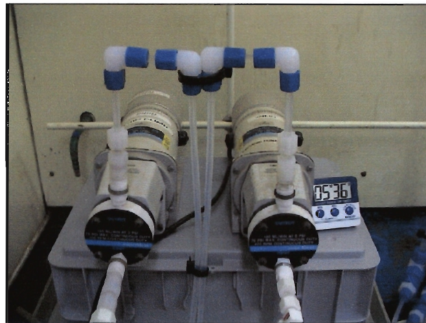
Figure 2-5 Masterflex metering pumps.
