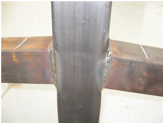
Fig. 39 Weld failure in a RHS X-joint
