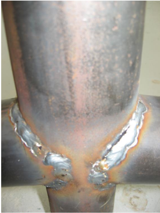
Fig. 37 Weld failure in CHS X-joint
