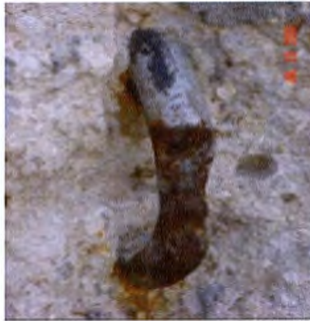
Figure 2.1: Pitting corrosion of reinforced concrete
