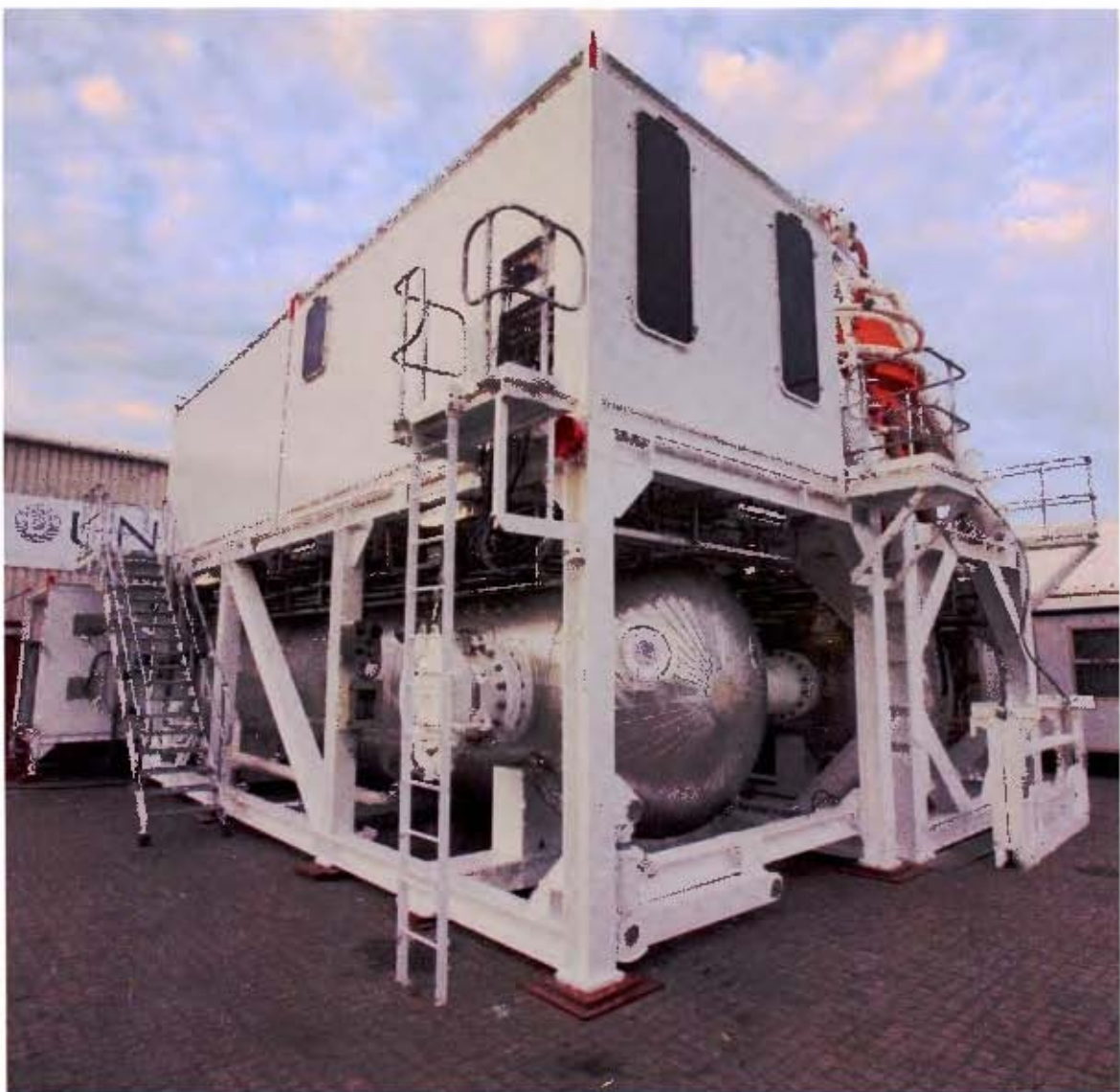
Figure 3.1 Picture · Hydra saturation dive system.
