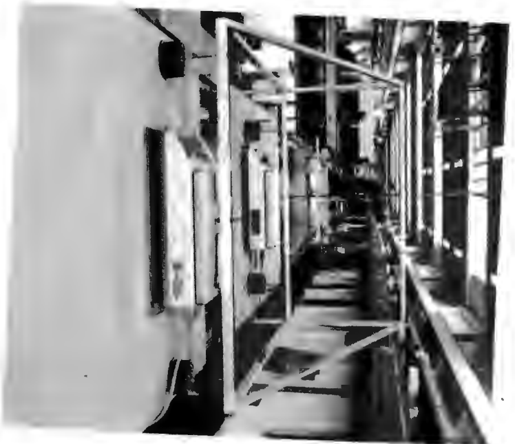
(b) Downstream view, showing four dashpots fixed to frame.
