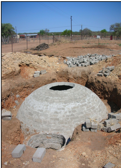
Figure 9 Photo: Rural digester Giyani, Limpopo, 15m 3 feedstock: cow manure (Authors own photo)
