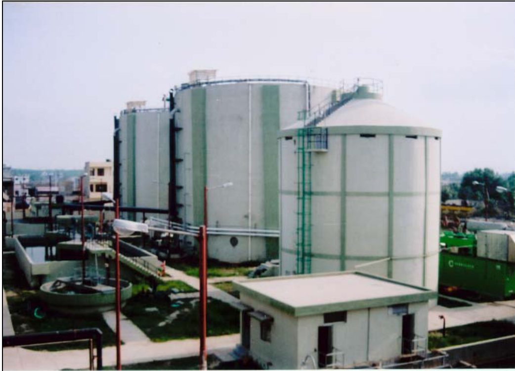
Figure 10 Photo of 1.0 MW power project based on cattle dung at Haebowal Dairy Complex Ludhiana, Punjab (Dhussa, 2004)
