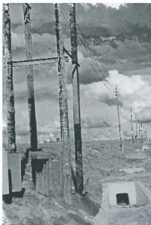
Pole-mounted transformer, emptied of oil.
