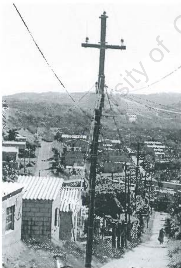
Bare MV conductors, LV abc on wood poles
