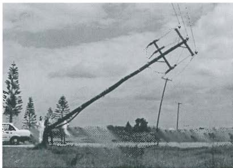
Figure 5-3: Low hanging conductor as a result of attempted cable and conductor theft by cutting two wood poles
