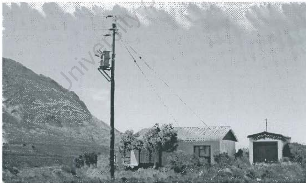
Figure 4-6: Typical three-phase small transformer installation with excess capacity
