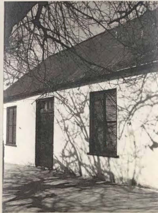
42,43. The Messenger's House at Grahamstown. Originally thatched, and (presumably) without louvred shutters.
