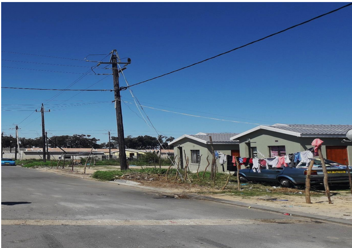
Figure 10: Residents tapping electricity directly from Eskom pole in RDP houses.
