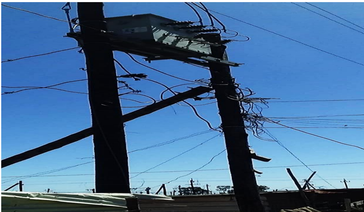
Figure 12: Residents connecting directly from Eskom transformers.
