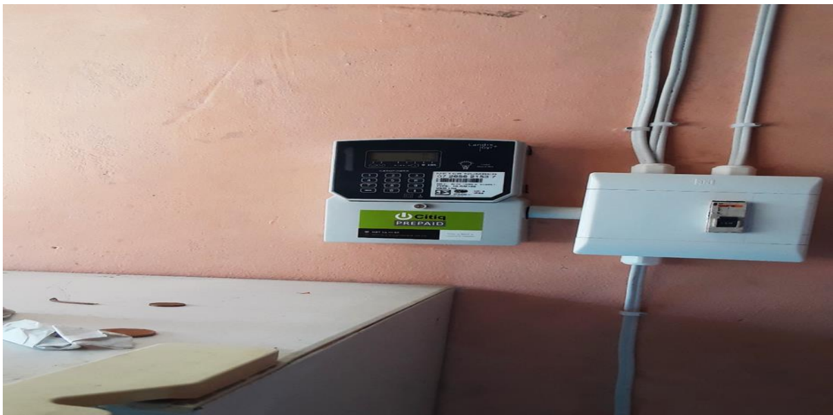
Figure 9: Fully installed Citiq electricity prepaid meter.
