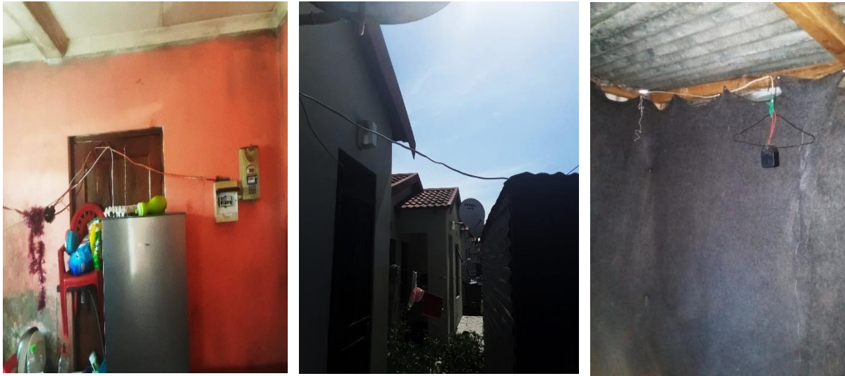
Figure 7: Electricity Extension between RDP and backyard house.
