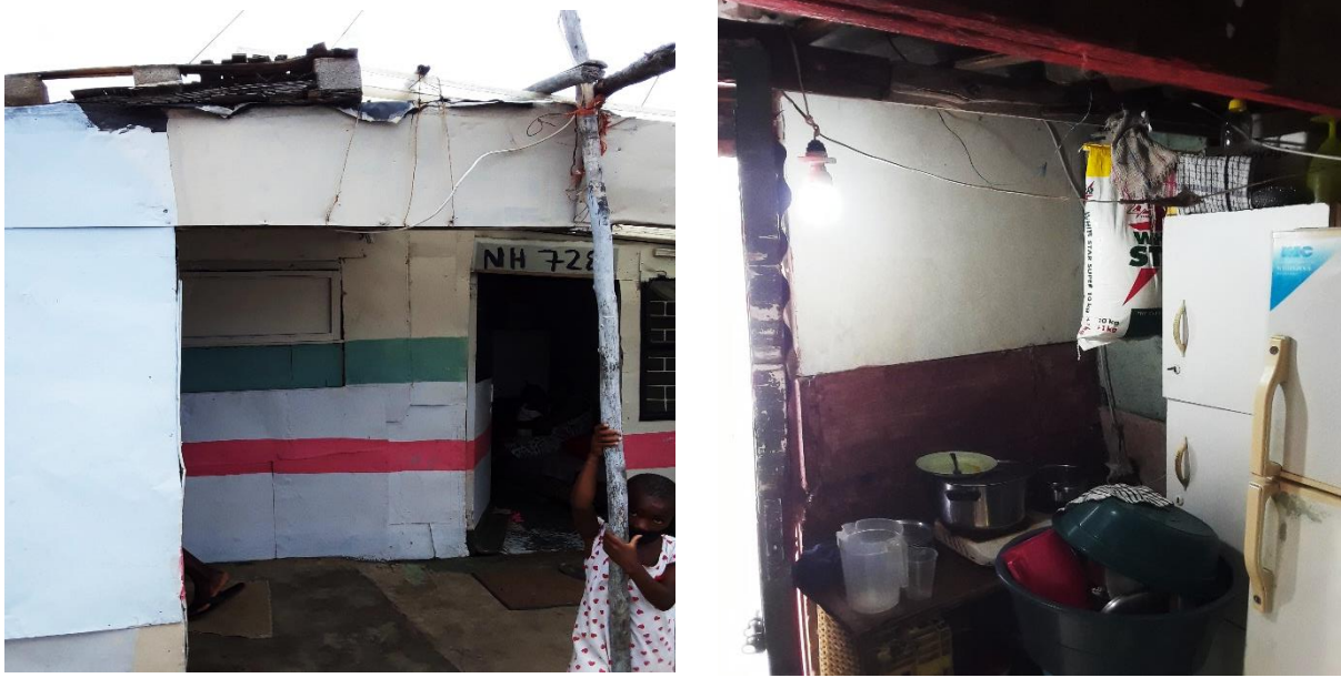
Figure 8: Electricity Extension between multiple rooms in Eskom electrified resident made houses.
