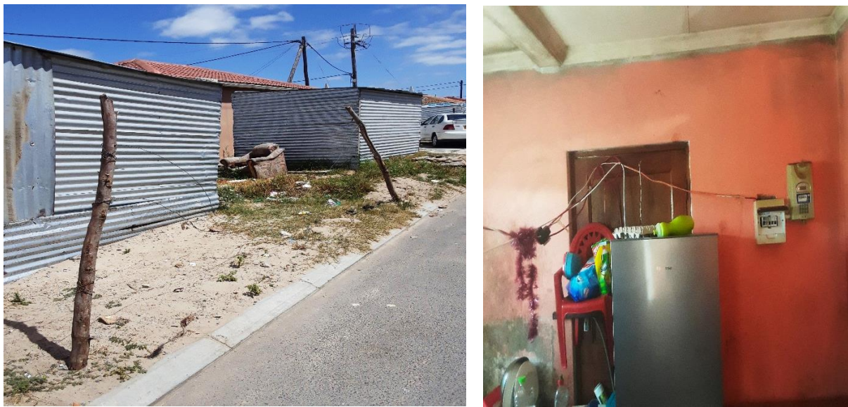
Figure 6: Electricity extensions to backyard houses.
