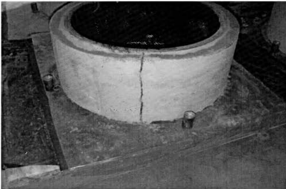
Figure 4.16: Typical crack in ring specimens.
