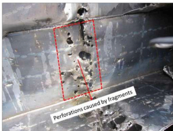
Figure 2.28: Perforation damage observed adjacent to charge location, as observed by Kong et al. [64]
