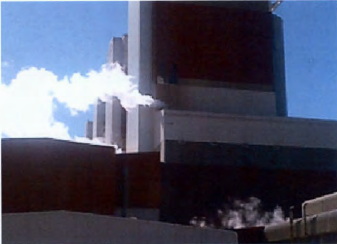
Figure 3: Steam loss due to internally leaking drain valves
