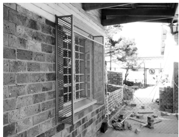
Figure 63 [right]: Siyazingisa Primary School, Gugulethu: Photograph to show retrofitting of windows with cage-like security bars
