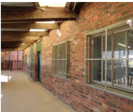
Figure 54: Wesbank No1 Primary School: The architects designed security screens over windows on the street facing façade only. Photograph to show how internal façades have been retrofitted with generic cage-like bars due to being perceived as vulnerable.
