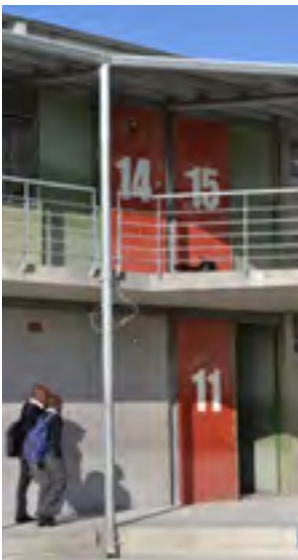
Figure 53: Usasazo Secondary School: Photograph to show barbed wire on downpipe to prevent people climbing the pipe to gain access to the upper level
