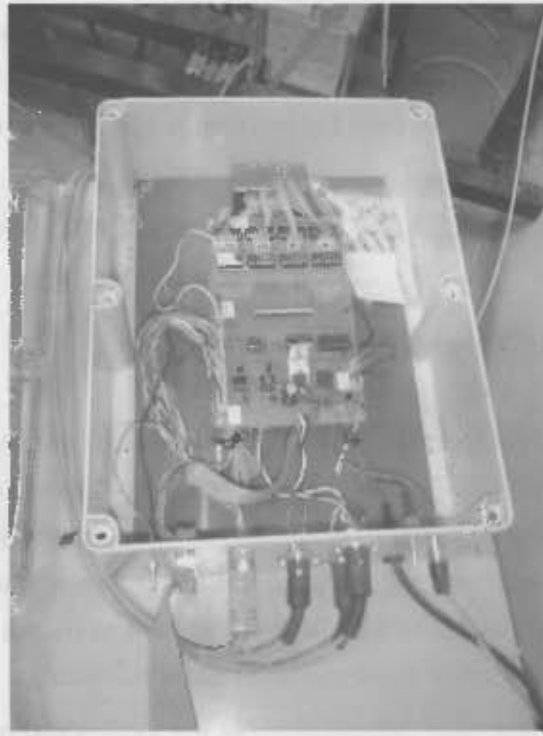
Figure 2.6: Photograph showing electronics box.
