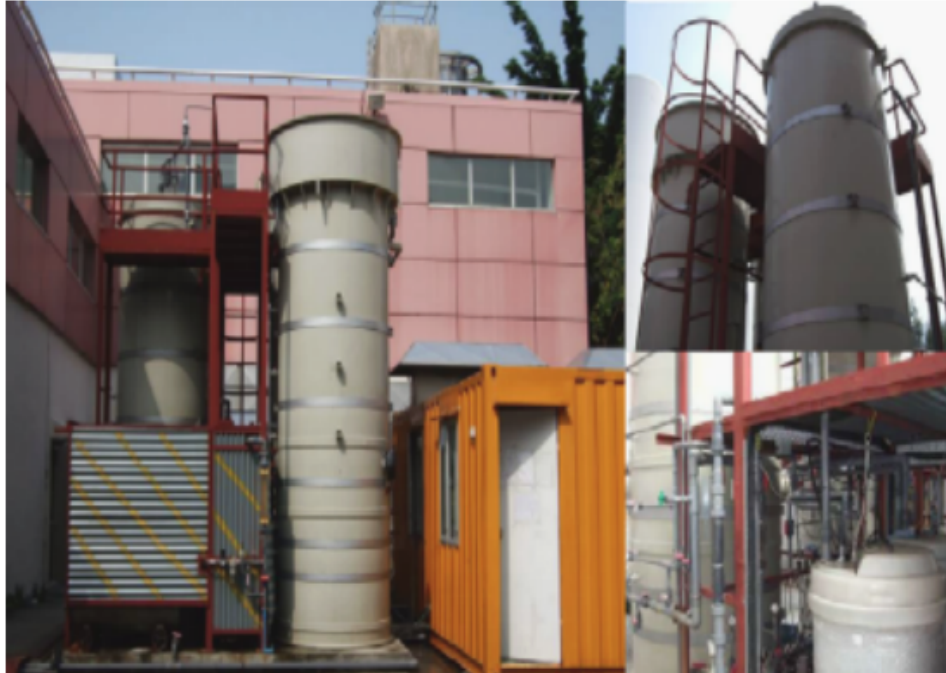
Figure 2.5 The SANI pilot facility was established at the Tung Chung Sewage Pump Station (TCSPS) in Hong Kong. 46
