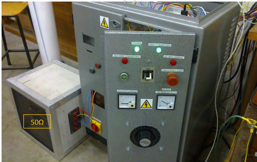
Figure 5.24: Experimental setup showing 50ohm load connected to each phase.
