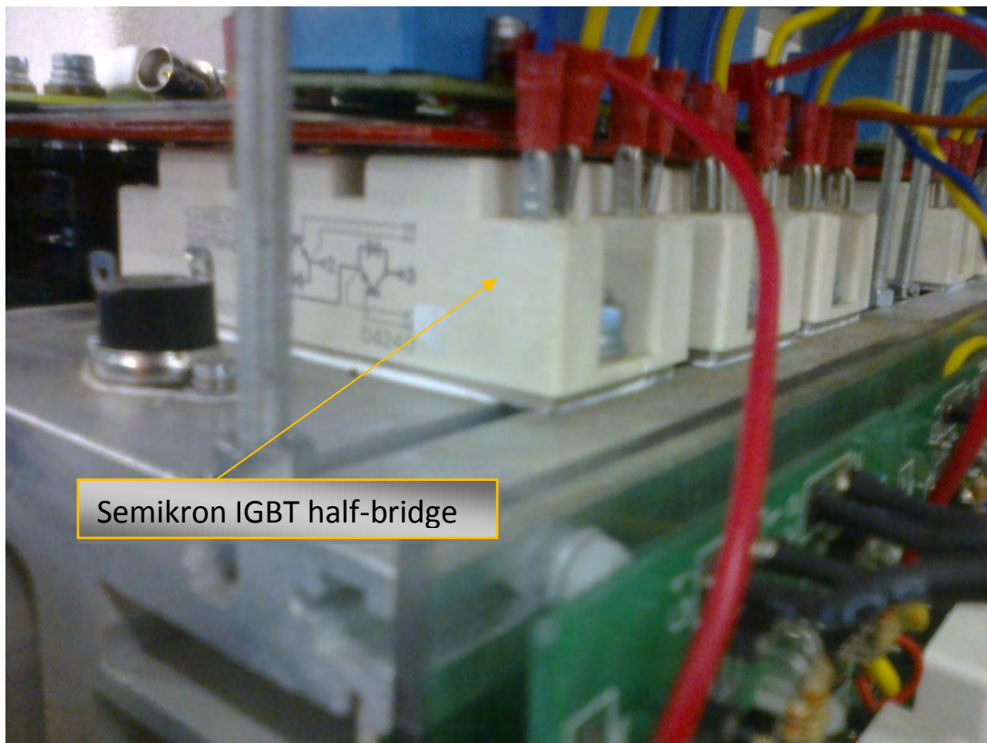
Figure 3.13: Semikron IGBT half-bridge mounted on heat sink of back to back converter
