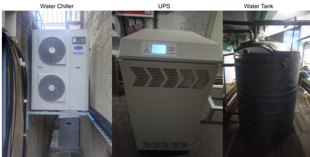
Figure 4.22: Shows the water chiller, ups and water tank.
