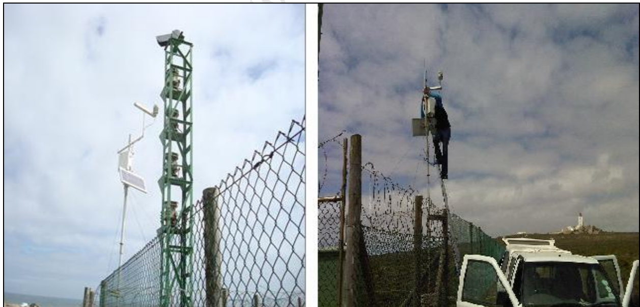
Figure 2.1: Figure showing an Automatic Weather Station installed along the foghorn with the Cape Columbine Lighthouse on the background as shown on the figure on the right.
