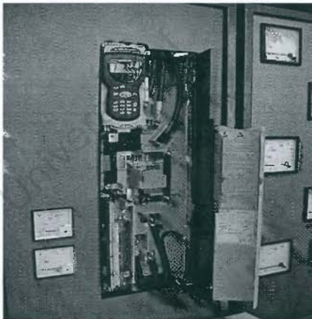
Figure 2.12: Induction motor, 75 kW VSD on the supply panel
