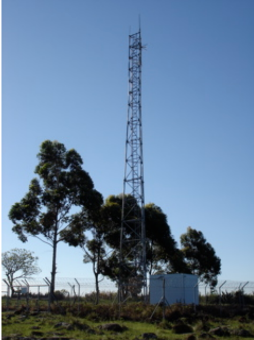
Figure D-4 Eskom tower relay station
