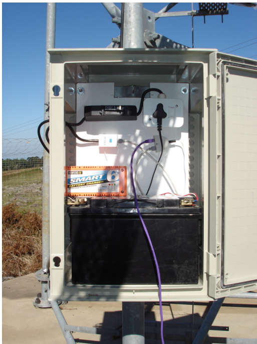
Figure 7-4 Battery enclosure at the Eskom tower relay
