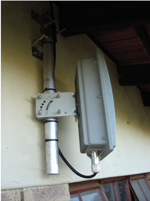
Figure 7-6 Waterproof enclosure mounted at Canzibe hospital
