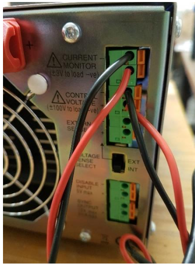
Figure 3-22: Current monitor connection and analogue control voltage connection to the load
