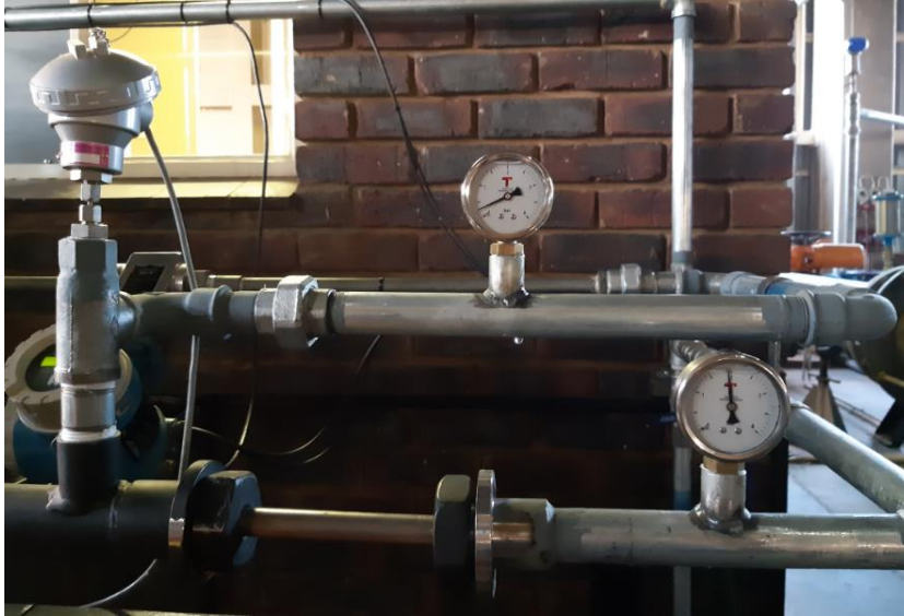
Figure 4-17: Installed Pressure gauges
