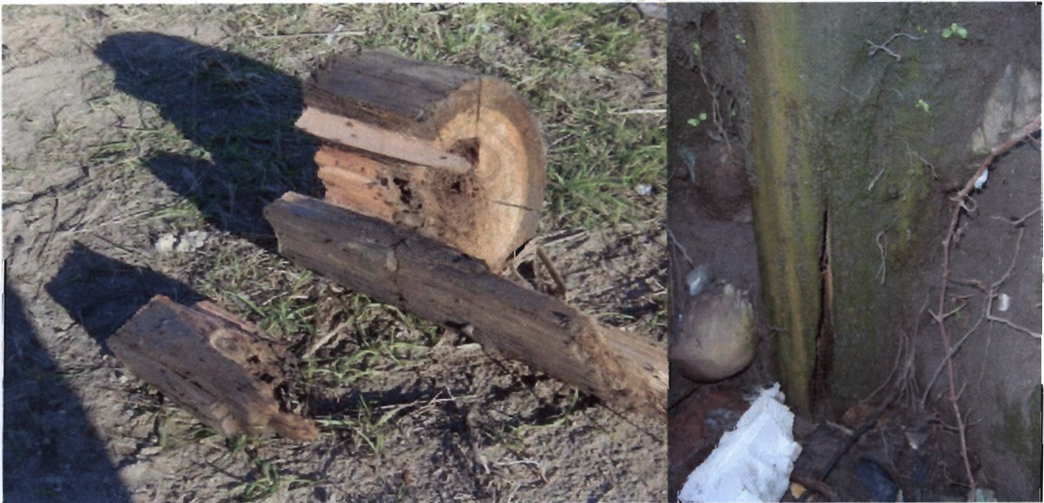
(a) Termite Damaged Pole
