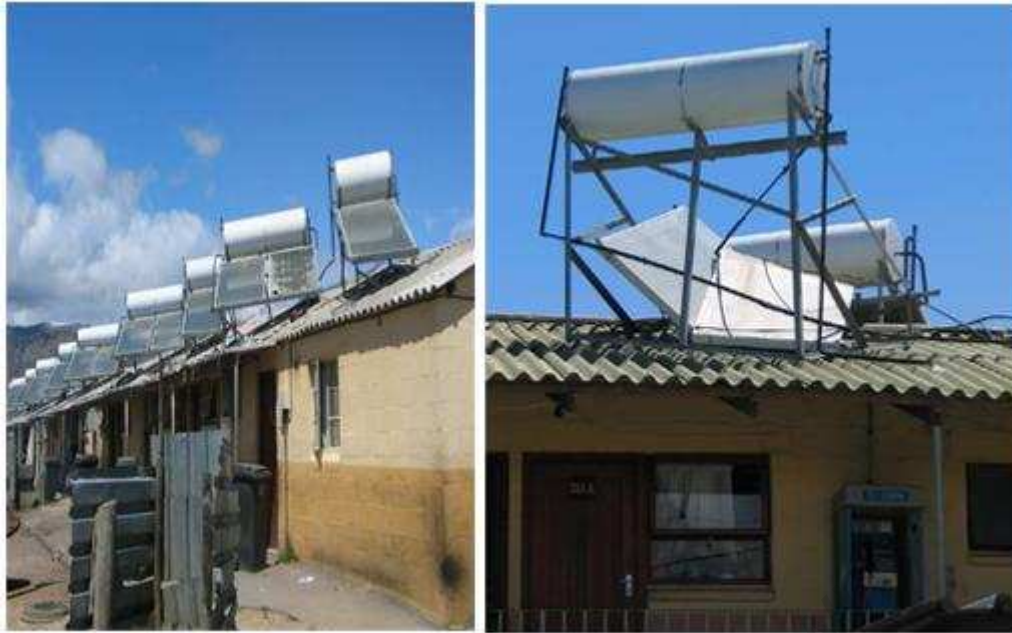
Figure 16. SWHs installed and not maintained
