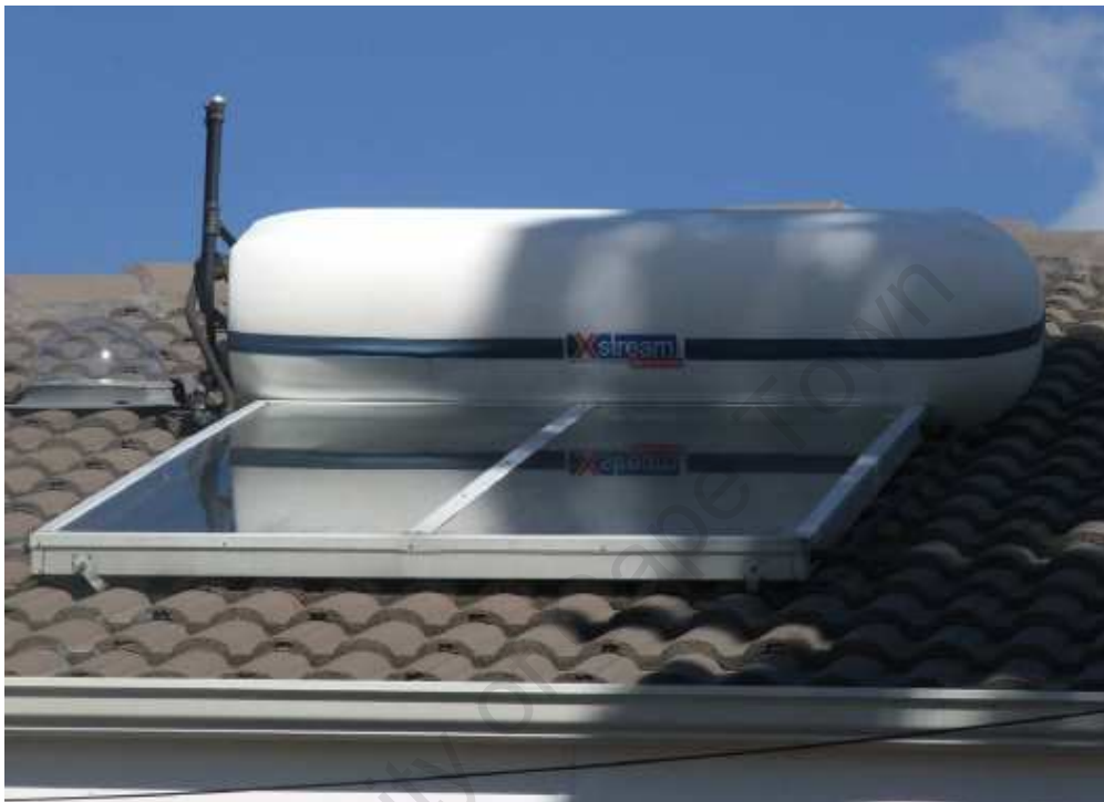
Figure 9. Typical flat plate SWH system
