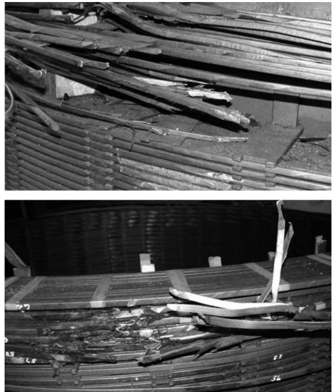
Fig. 2. Windings of Eskom transformers presumed damaged by the geomagnetic storm on 29 October 2003.
