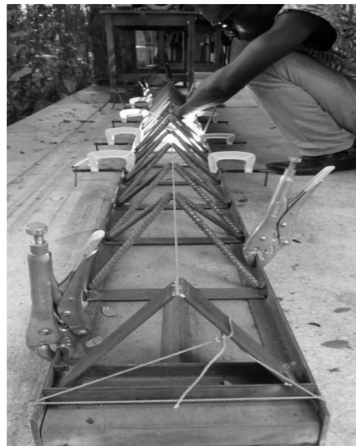
Construction of Semi-Octet Truss uploaded to website by AMP team Images Sourced from https://qamp.net/tag/welding/ , accessed 6 April 2022
