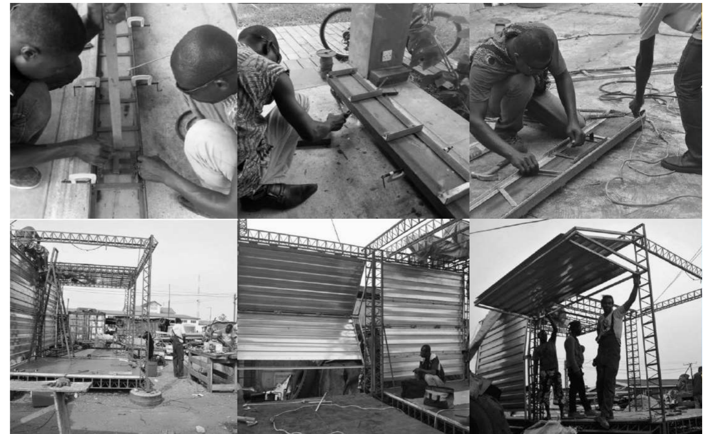
Collage of Construction process By Author Images Sourced from https://qamp.net/tag/welding/ , accessed 6 April 2022
