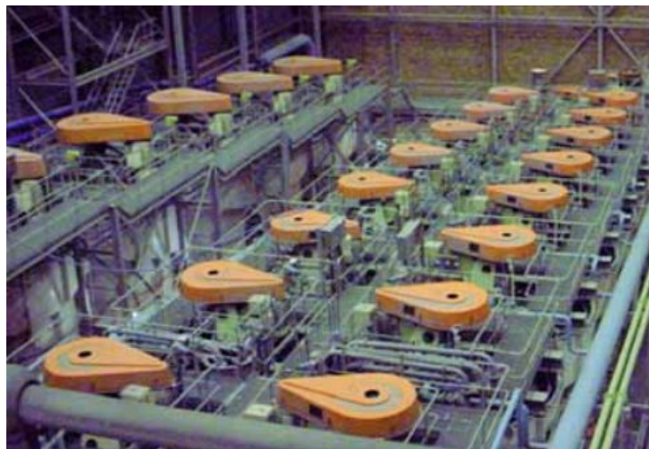
Figure 2.3.: Three flotation banks in an industrial flotation plant.
