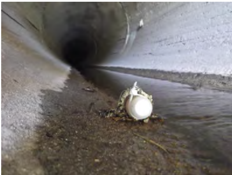
Figure 3.2: The wire holder securing the iButton in the Stormwater pipe outlet
