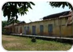
Saaman JHS building with roofrazed off
