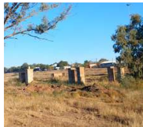
Broken Bridge over the Prieska river (Flood plain)
