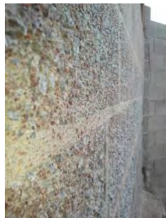
Figure 110: Eroded surface of concrete block boundary wall oyster production company (Author, 2013)
