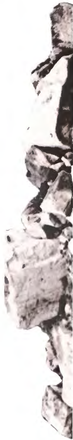
Figure 42: South facing wall, showing granite intrusion
