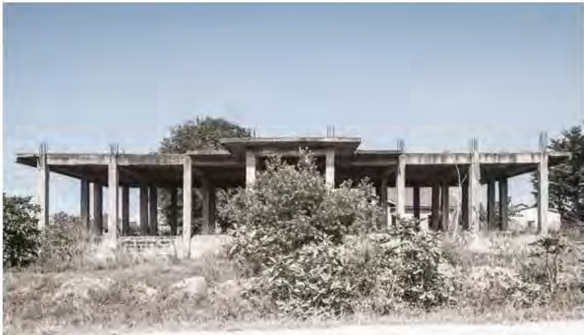
Roadside indigenous overgrowth along Mrisho Kikwete Drive. Abandoned residential structure. The road is named after the President of Tanzania Ukuni, Bagamoyo, 27 September 2016
