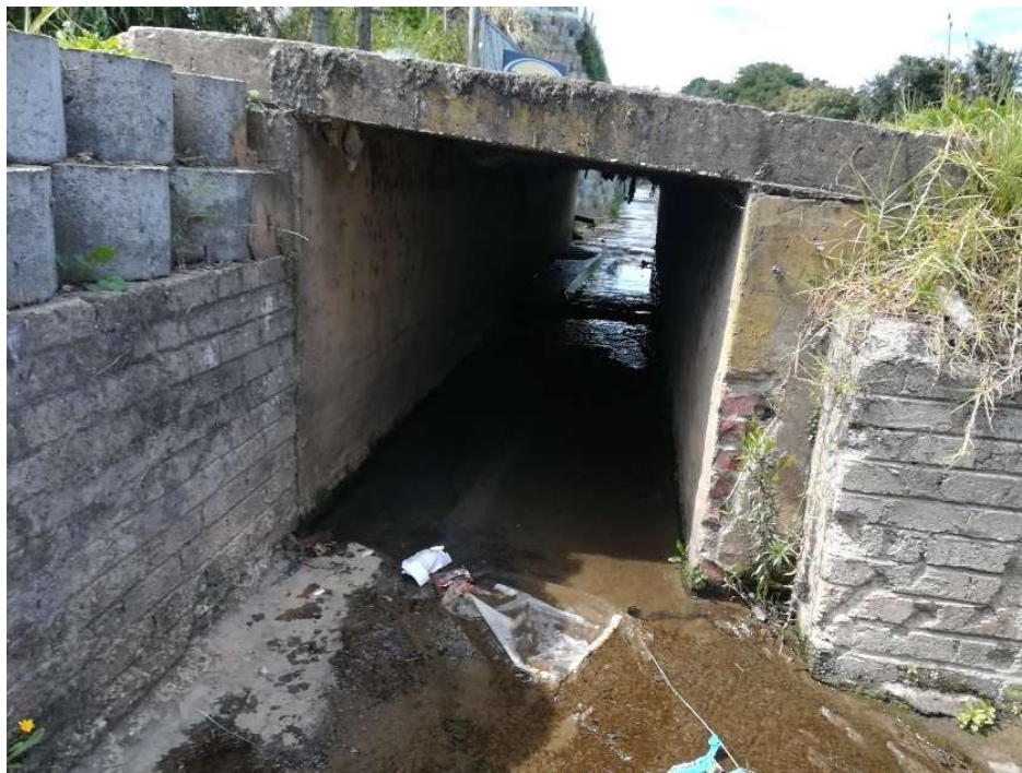
Figure 3-18: Vigilance Drive Drain water level monitoring point 4a
