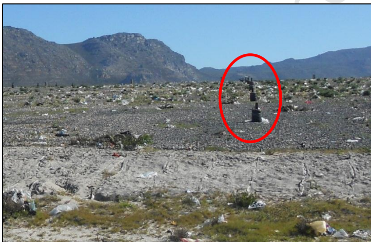
Figure 6: Gas pipes at Coastal Park Landfill
