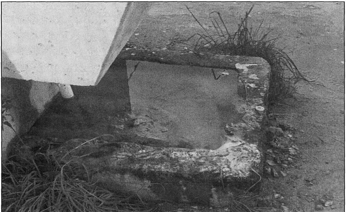
Picture 4.1: Sewage overflowing from the gulleys below the washbasin
