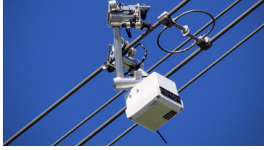
Figure 1.6: UKZN's power line robot [6].
