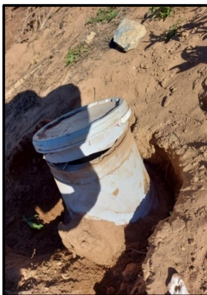
Figure 6-16: Deployment 0 - System Vandalised
