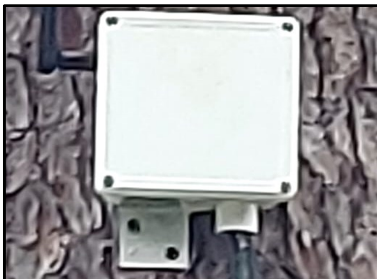
Figure 4-21: Weatherproof Enclosure with L-bracket Housing the Sensor Nodes
