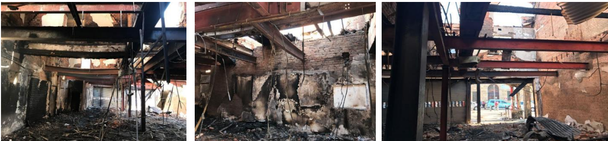
FIGURE 19: Images of building in CBD burnt during 2021 civil unrest
