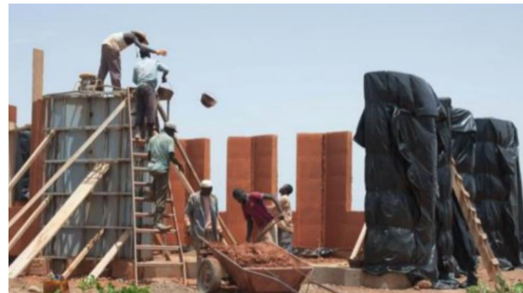
FIGURE 34: Cast In-Situ Clay Walls Being Mixed and Poured on Site by Local Community Members
