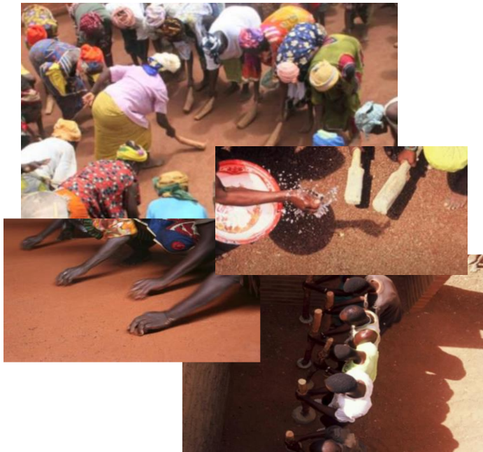
FIGURE 36: Local Men and Women Using Their Feet, Water and Traditional Tools to Compress And Stamp The Clay Flooring
