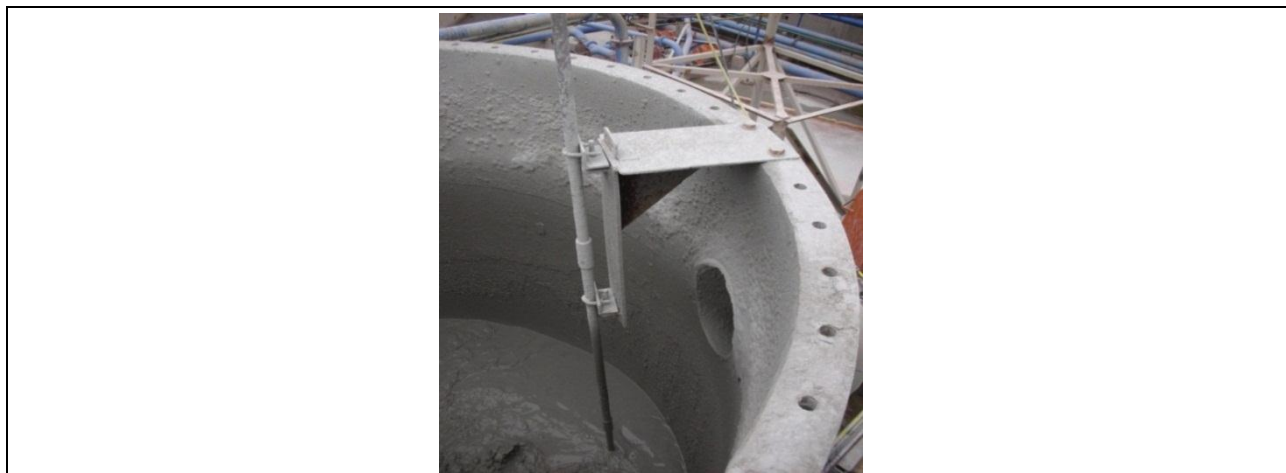
Figure 7.2 Stainless steel filter probe in residue sump
