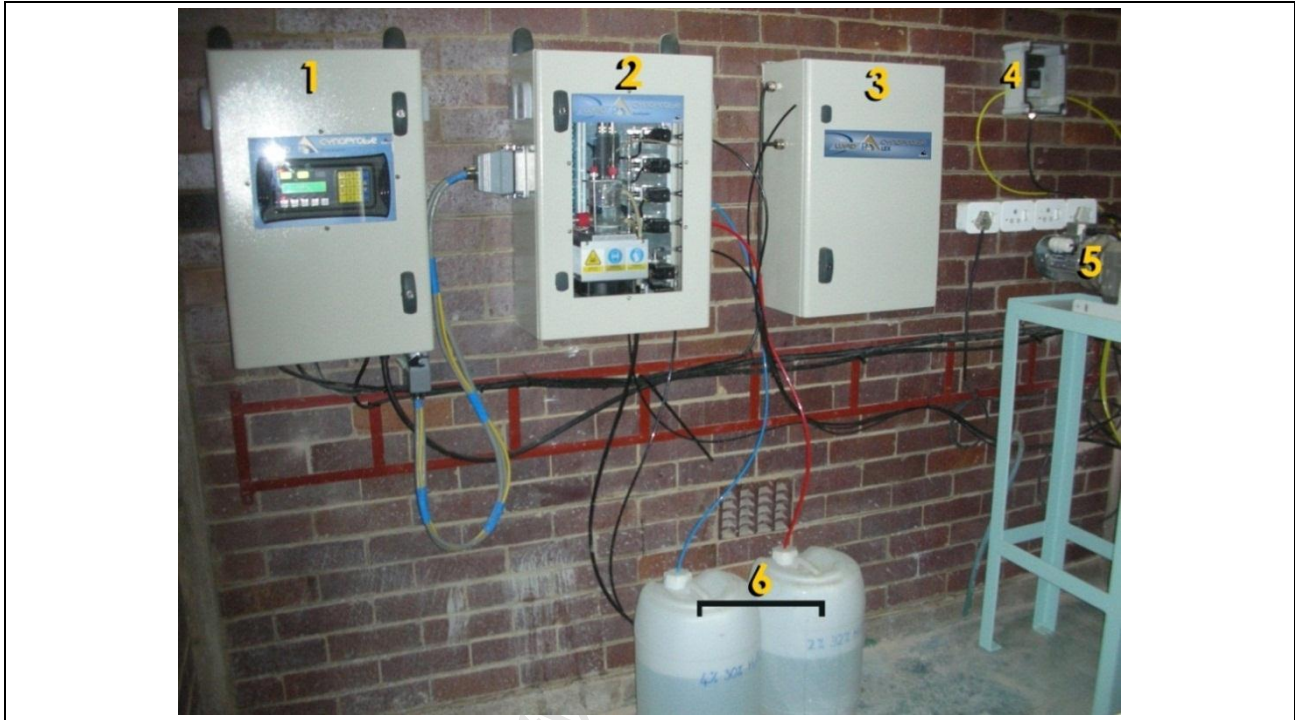
Figure 7.1 A local Cynoprobe installation in the CIP residue section
