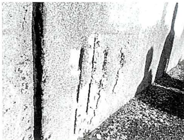
Figure 37: De Waal road bridge showing signs of concrete spalling and rebar corrosion with inadequate concrete cover. (taken 2016)
