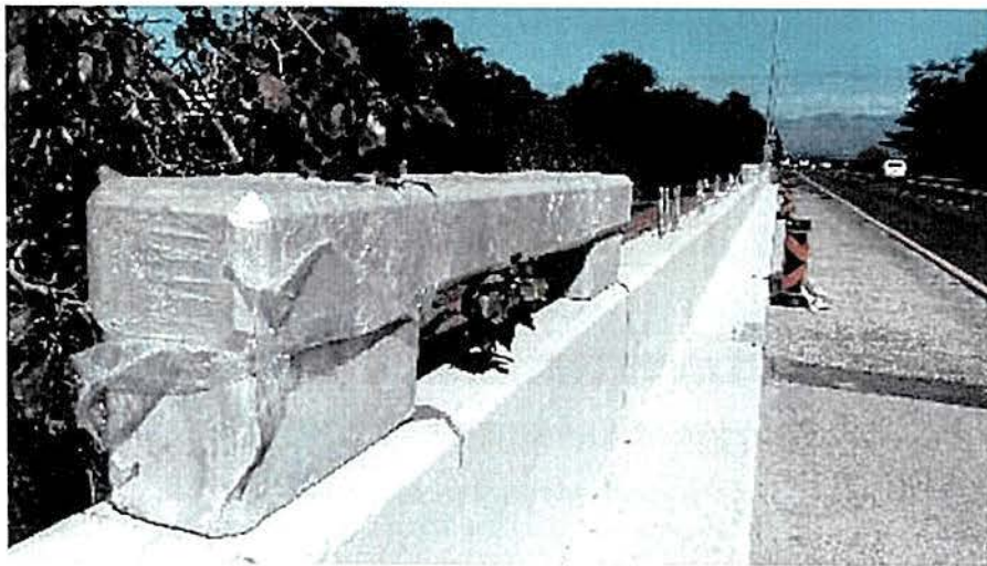
Figure 38: A precast concrete handrail delivered and installed on site. The handrails are steam cured and wrapped in plastic before delivery to site.
