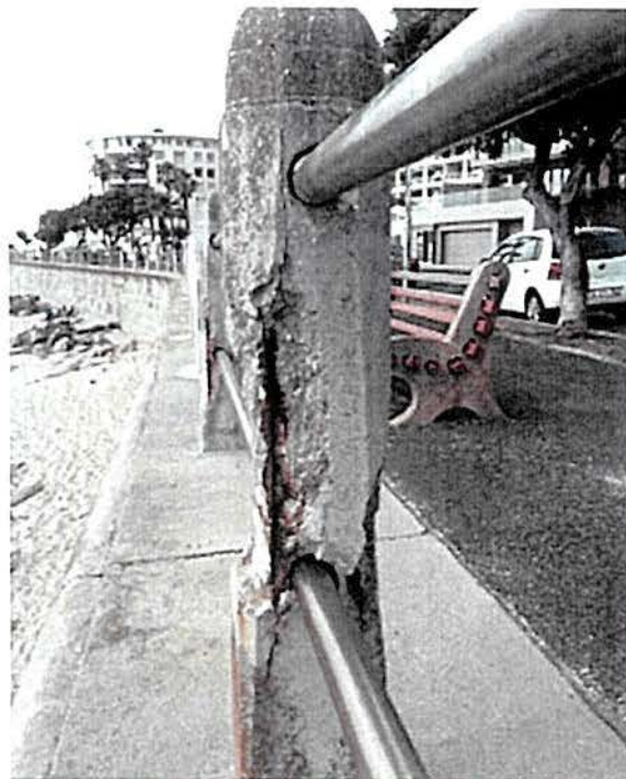
Figure 36: Rebar corrosion of a bollard on the sea point sea wall. (2016)
