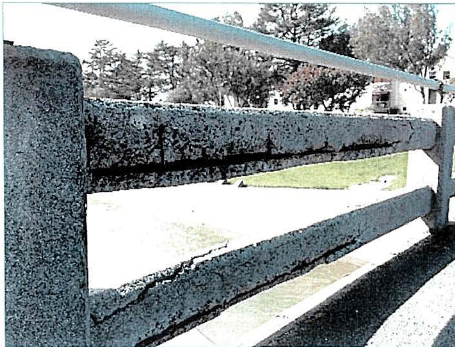
Figure 2 : Concrete deterioration and damage takes place in the form of spalling of the concrete cover and steel corrosion in Pinelands, Cape Town. The cracks normally develop above the steel and as the corrosion progresses the cover concrete is detached. In this case the deterioration was caused by low concrete cover and porosity concrete.
