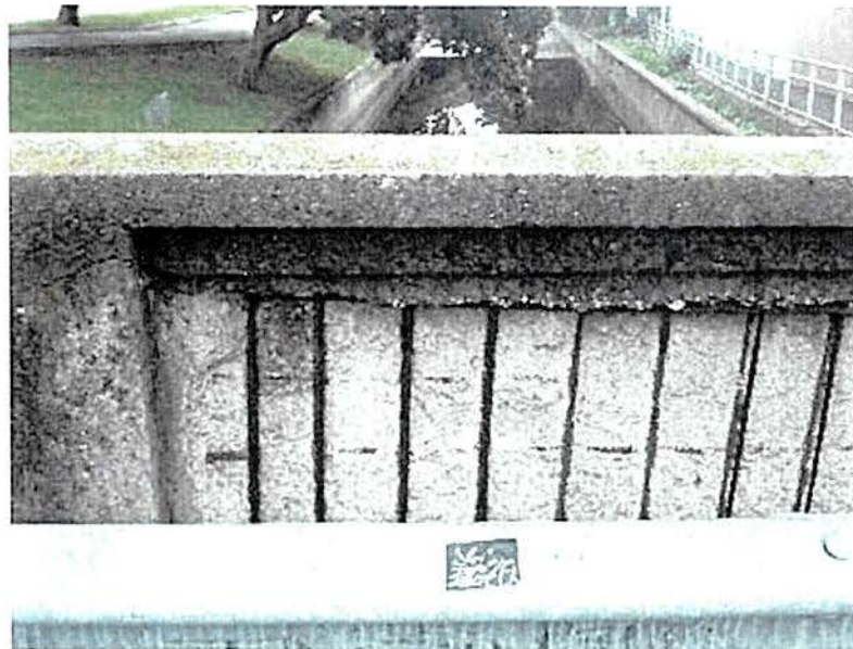
Figure 39: Extensive concrete spalling on existing concrete balustrade of Alma Road Bridge (Fatima Adams, July 2016)
