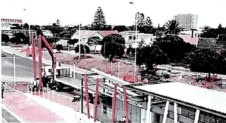
Figure 43: Concrete used for the bus way and the bus stations (City of Cape Town , 2007)
