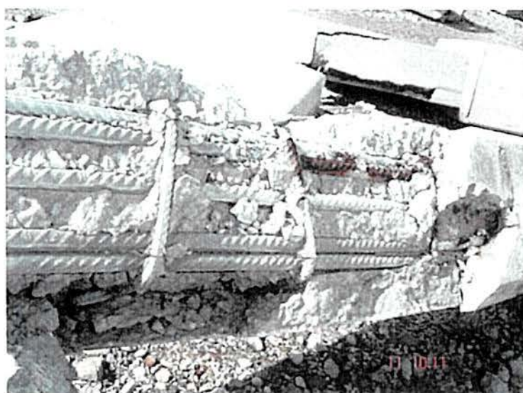
Figure 15 Isolated rust in regions of minimal concrete cover. (HDGASA, 2015)
