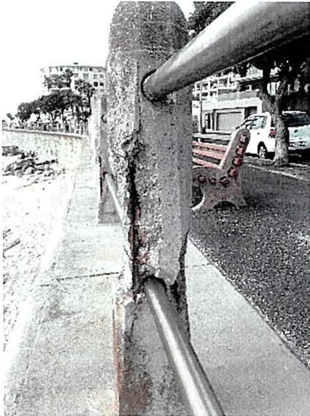
Figure 4: Concrete bollard located on the Atlantic Seaboard in a Spray Zone. The Concrete bollard shows heavy corrosion damage on the coast of Sea Point (Taken Oct 2016)
