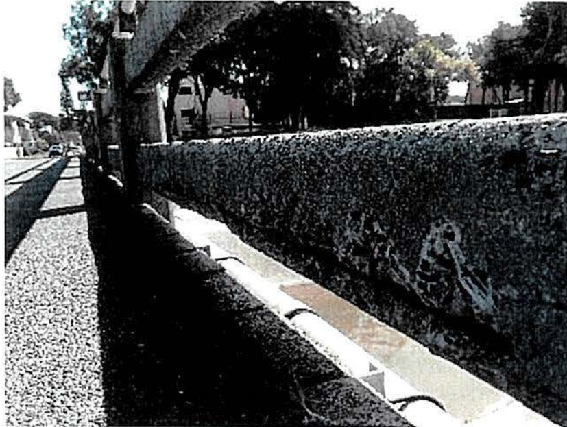
Figure 5. Pinelands road bridge spalling and rebar corrosion. Taken September 2016
