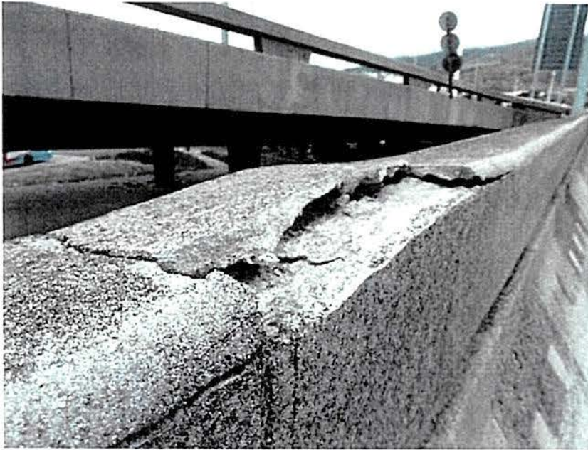
Figure 41: Concrete spalling on existing balustrade of the Foreshore Freeways, Cape Town (2015)
