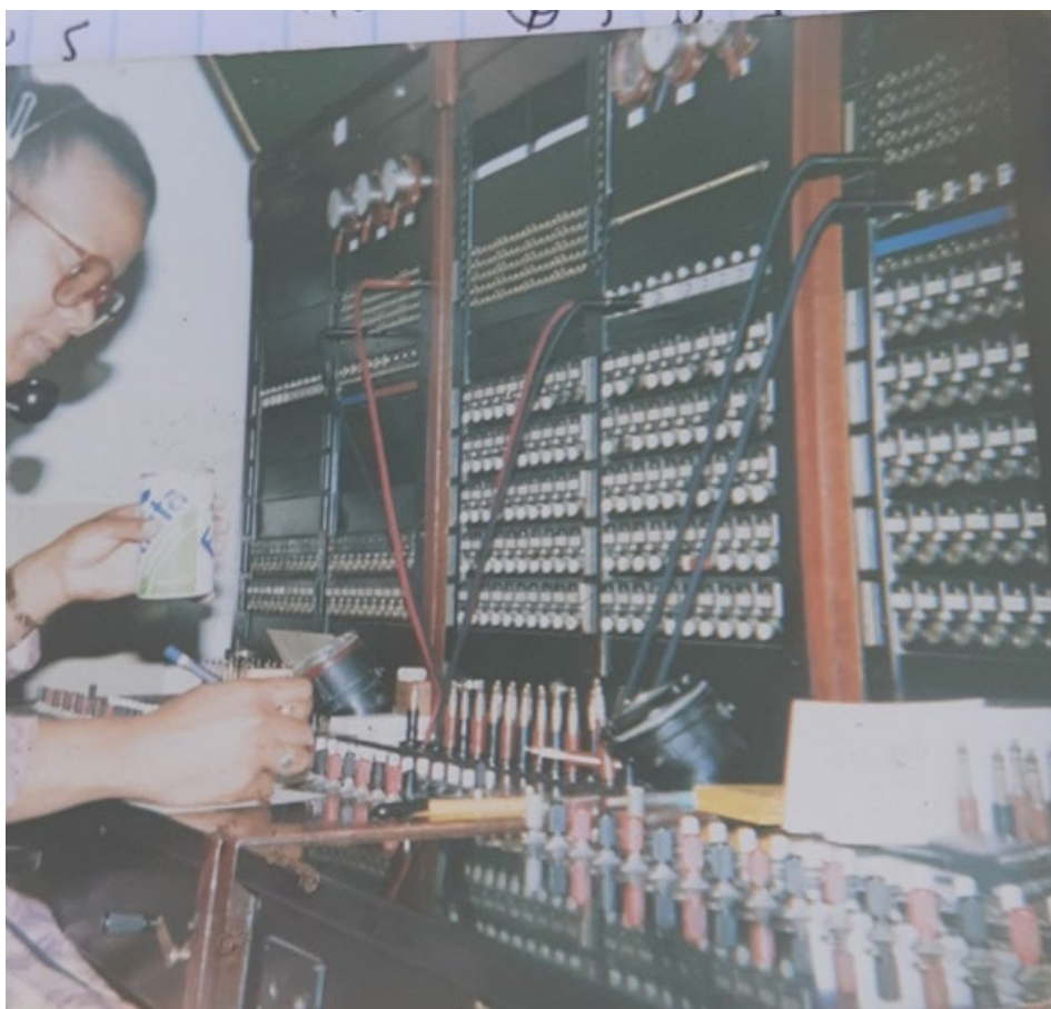
Figure 6.8 An image of telephone exchange unit at the old Haarlem Post Office. Photo credit: Geraldine Wildeman’s photo album (9 June 2021).
