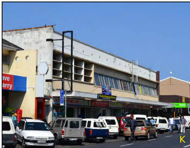
Figure 5.17 Dilapidated building along Durban Road
