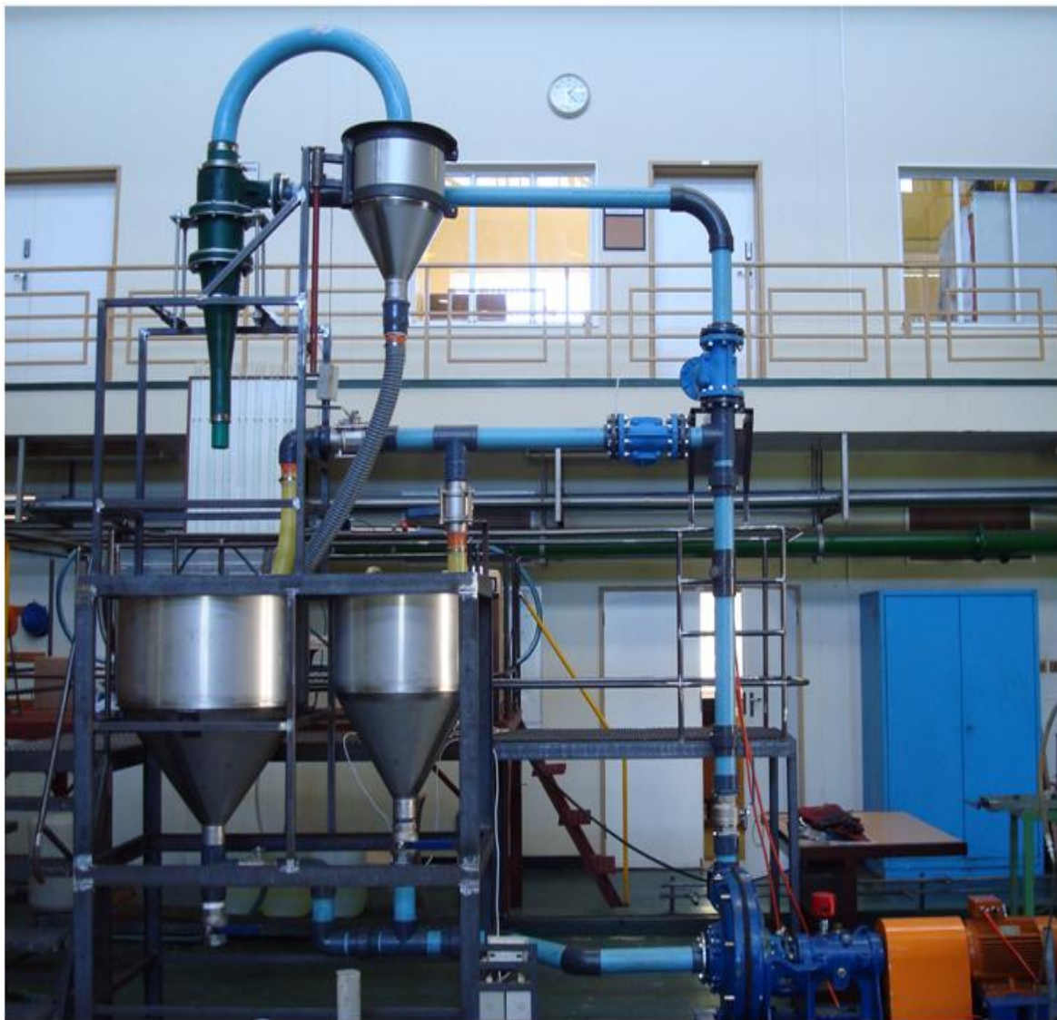
Figure 4-19. 165 mm hydrocyclone test rig
