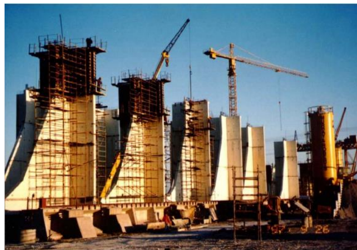
Figure 2-2: Precast counterfort wall units under construction in Saldanha Bay, South Africa (Paul & Zietman, 1999:11).
