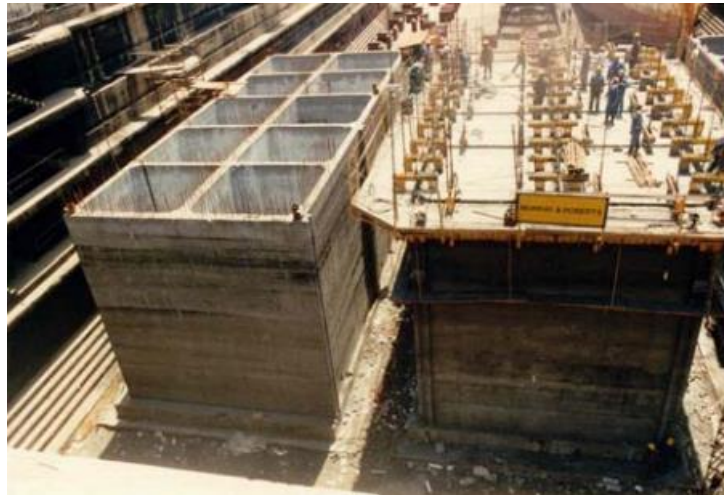
Figure 2-1: Two caisson units under construction in the Port of Cape Town (Smith, 2016b:23).
