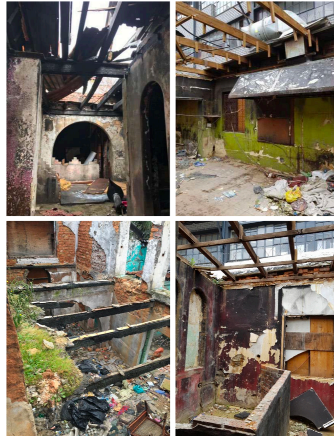
FIGURES 75 - 78 : Photographs showing ruined state of the interior of the building
