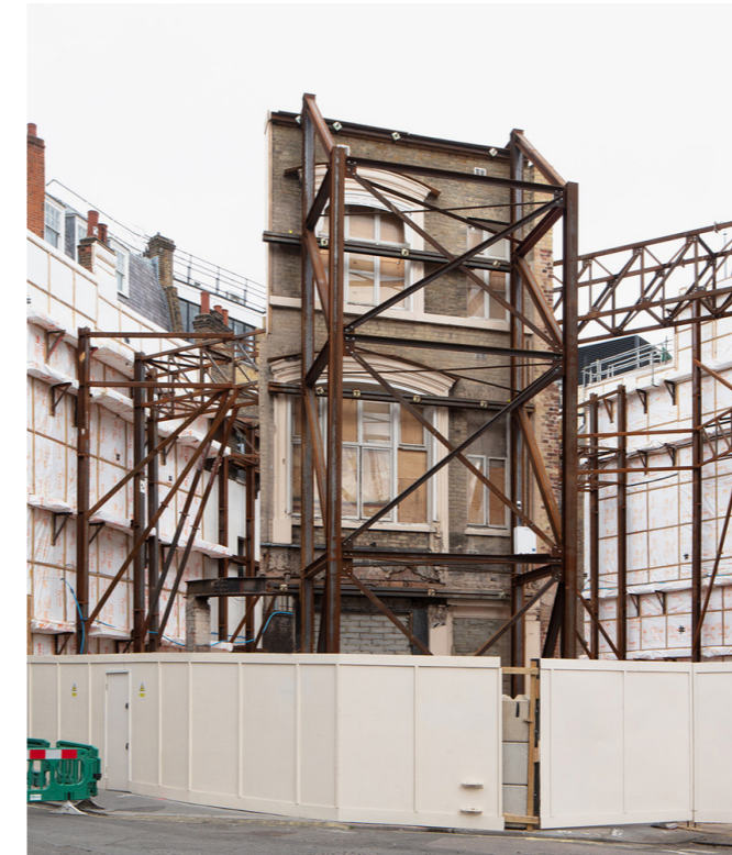
FIGURE 89 : Historical Facade Retention using a steel frame system. Sometimes, simple scaffolding or a wood frame is used, depending on the weight of the structure and recommendation by the engineer
