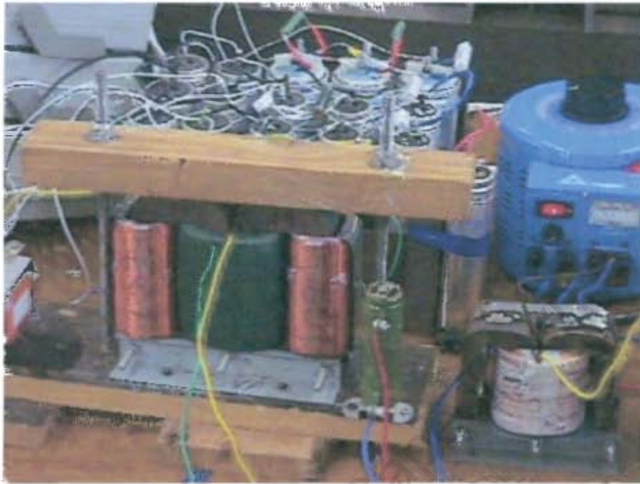
Fig: 7.50 Saturable reactor
